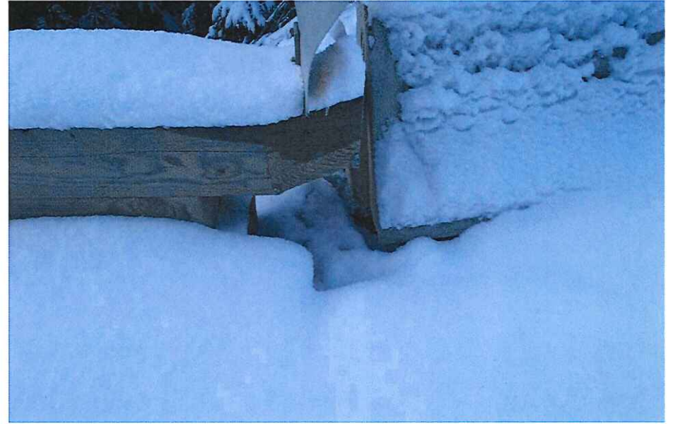
CK2360 Damaged guard rail
